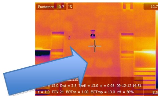
Figure 6: Example of structural damage discovered by a radiometric image that is invisible with a standard camera shot.
