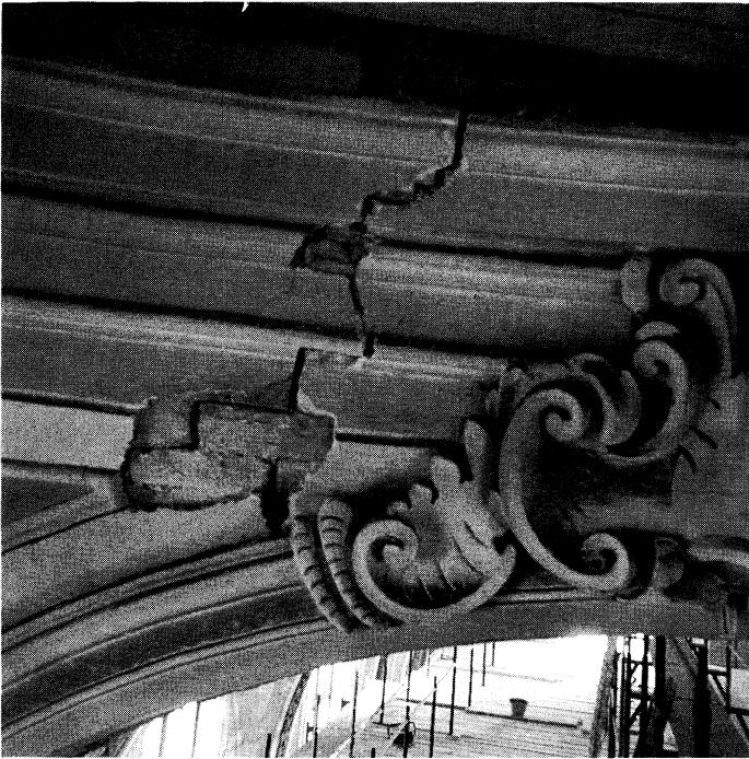
FIG. 1 : Damaged arche before intervention.
