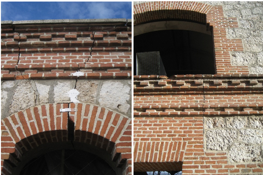
Figure 5: Images of some of the existing cracks on the façade load bearing walls.
