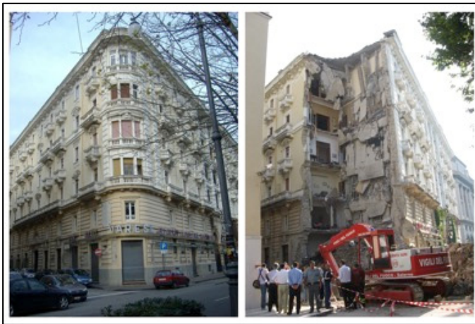
Figure 2: Picture of the south-west corner (between Verdi Street and Trieste Promenade) before (left) and after (right) the collapse.
