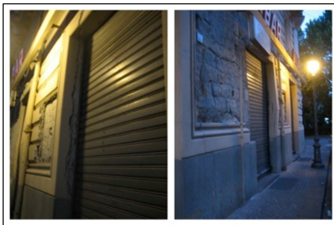
Figure 3: Cracks around two openings of the Varese Bar (Verdi Street, June 13, 2007).
