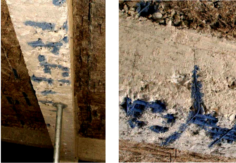
Figure 5: Local failures of a girder after plaster removal.
