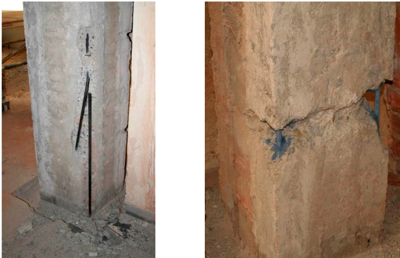
Figure 6: Local failures of a column after plaster removal.
