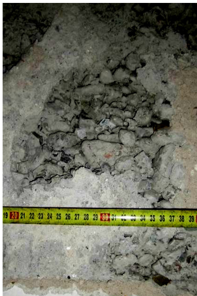
Figure 7: Faces of some columns after plaster removal.
