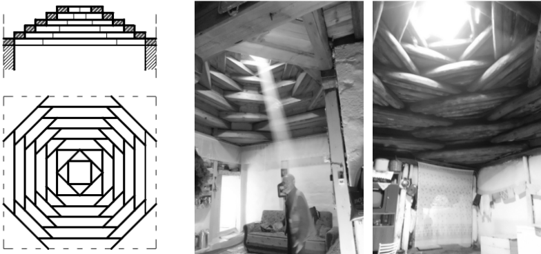
Figure 2: The section and plan of ‘ kırlangıç örtü ’ [7], and its interior view from dwellers’ houses who maintained it; the example of rectangular shaped timber elements (in the middle), and the example of round timber elements (on the right), both use the space as their living room (photos taken by the author).
