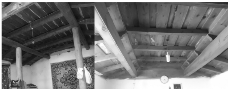
Figure 9: The interior view of a maintained roof with round timber elements, on the left; an example of renewed roof with rectangular timber, on the right (photos taken by the author).
