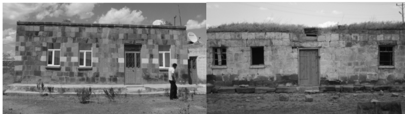
Figure 8: The exterior view of a maintained house with cut-stone wall, on the left; an unoccupied house with cut-stone wall, on the right (photos taken by the author).
