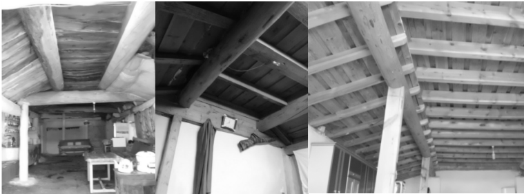
Figure 6: The interior views of round timber used for roof, the left and middle; an example of renewed rectangular shaped timber for roof from a dweller’s house (photos taken by the author).
