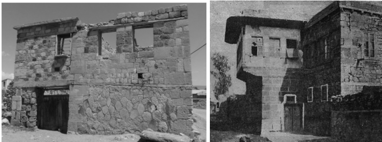
Figure 4: The exterior wall of a traditional house, which is a ruin today, on the left (photos taken by the author), and an old picture of these traditional architectural heritage from the year of 1947, on the right [8].
