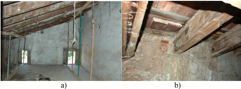
Figure 4: a) General view of the roof structure, b) a detail of the roof structure.
