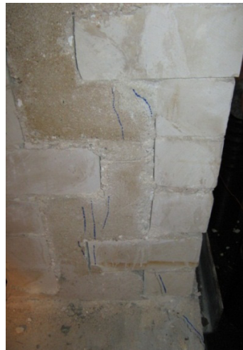
Crack initiation in W12
