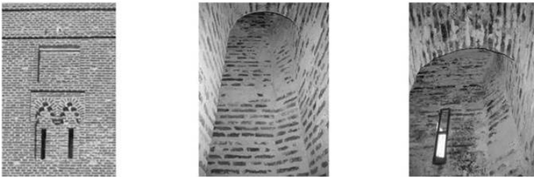
Figure 2: Aspects of the irregular mortar-brick disposition.
