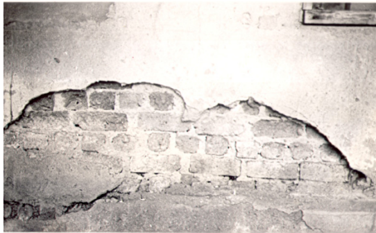
Figure 9: Broken wall plaster, revealing adobe brick core.
