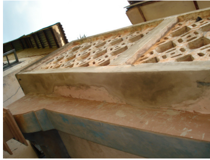
Figure 6: Adequate cement cover has been provided for the formerly exposed iron rods.
