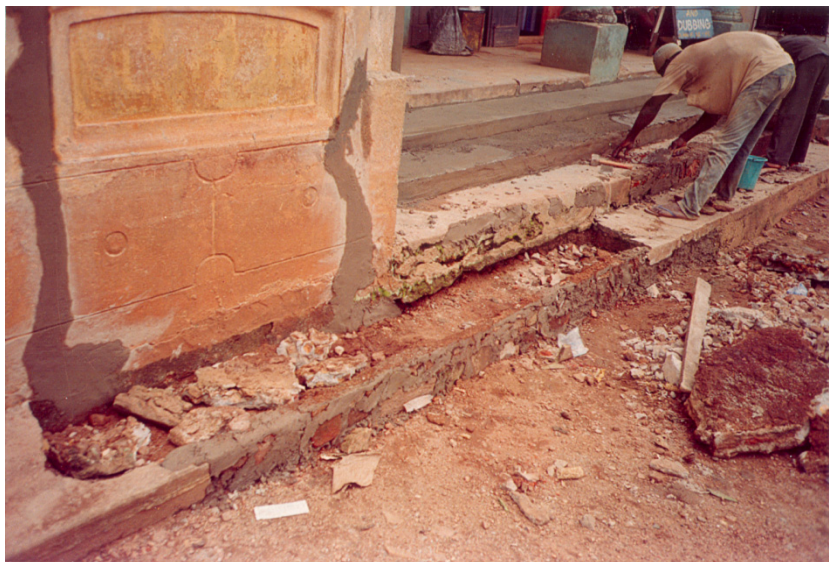
Figure 11: Repair-work to the badly-chipped entrance steps and cracks in the façade of the Ologbenla House, Moore Street, Ile-Ife.
