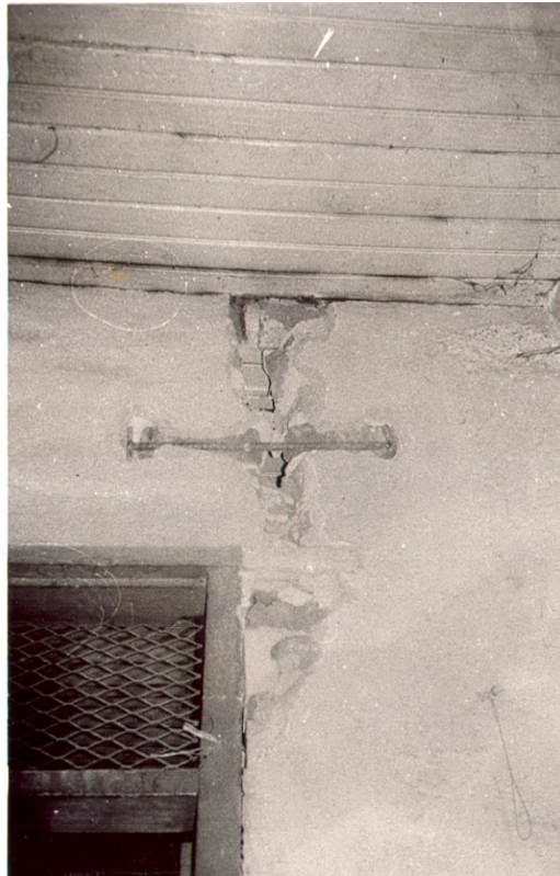
Figure 10: Major vertical crack, from right under the ceiling. A 12mm iron rod is embedded as bracing before the crack is sealed.
