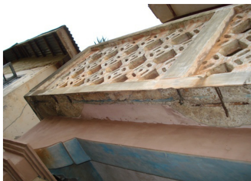
Figure 5: Iron reinforcement exposed to rust on underside of balcony.
