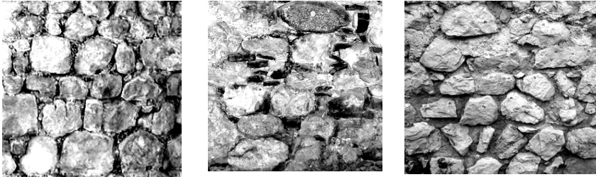
Figure 11: Masonry textures of the external walls, of the partition walls and of the Mastio.
