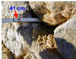
Figure 17: Inspection, which indicates the presence of a void.
