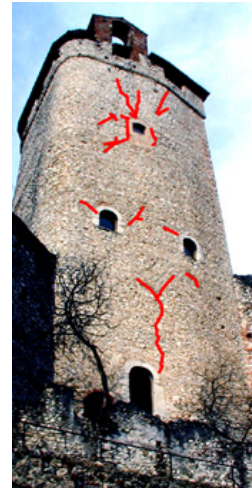
Figure 10: Crack pattern of the Mastio.
