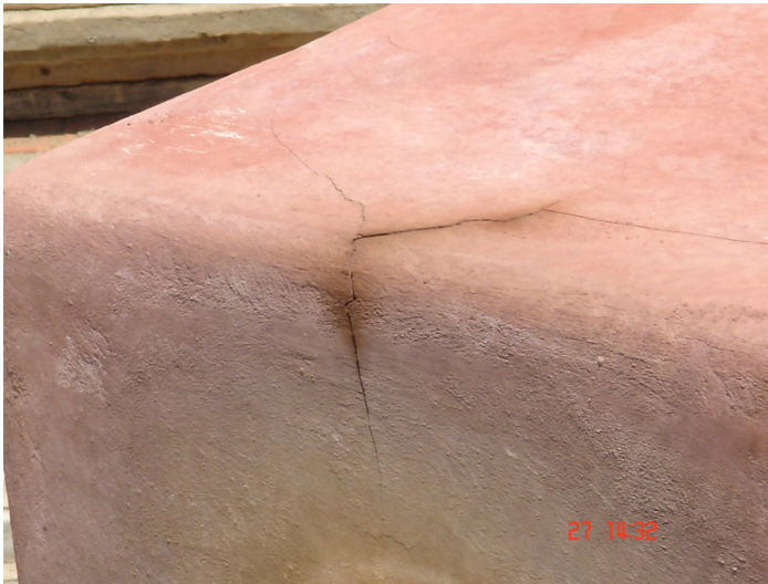
Figure 4: The increase in the crack width in specimen of Mix C after 1 hour.
