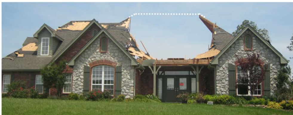
Figure 3: Failure of steep-sloping, stick-frame hip roof including removal of the largest faces. (Source: Stevenson [14] and Dr. D.O. Prevatt.)
