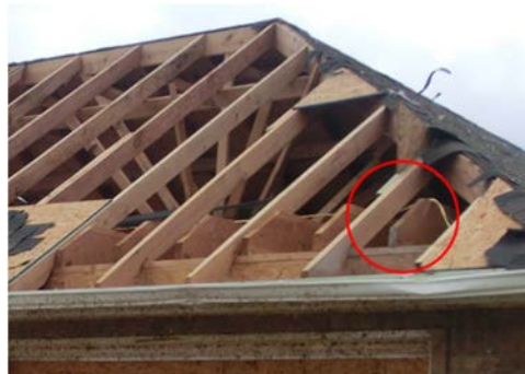
Figure 7: Intact stick-frame structure showing lack of connection between the jack rafter and ceiling joist. (Source: Dr. D.O. Prevatt.)
