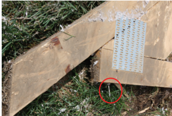
Figure 2: Failed RTWC with a single toe-nail, rather than three as required by the NBCC [10]. (Source: Kopp et al. [12].)
