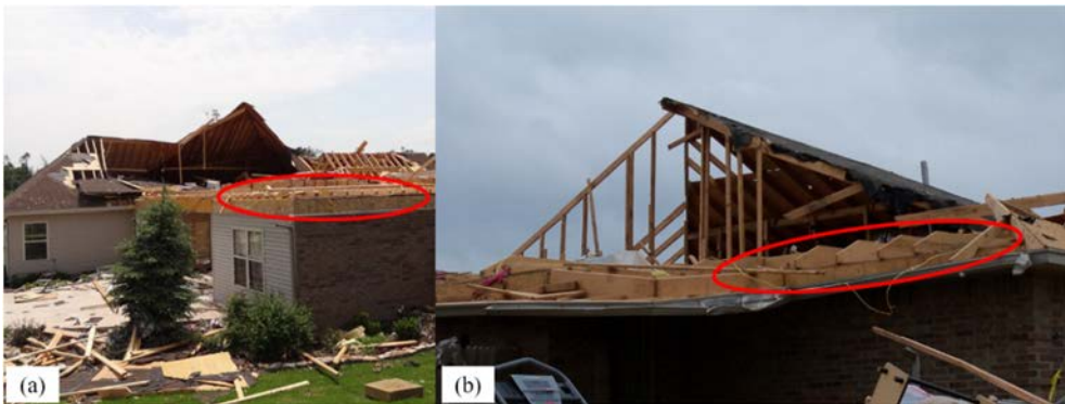
Figure 6: Framing failures in stick-frame hip roofs with intact ceiling joists. (Source: Dr. D.O. Prevatt.)
