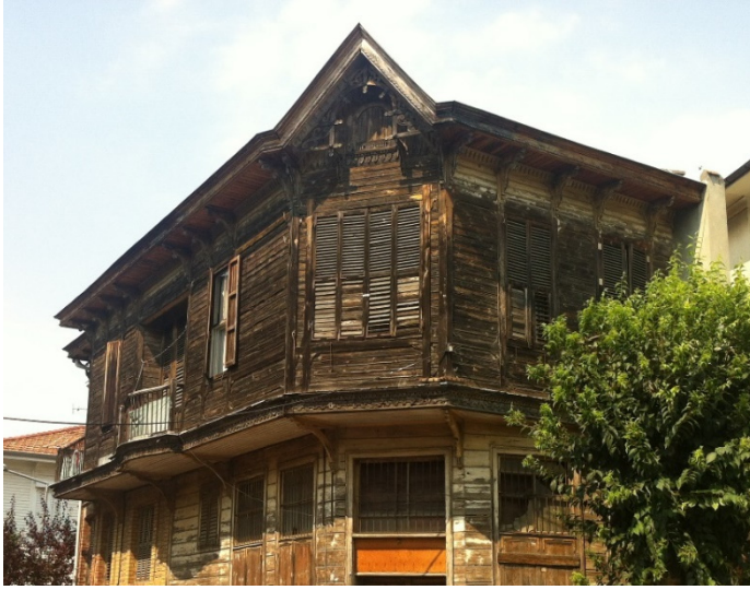
Figure 5: Steep pitch as a part of decoration of the façade.
