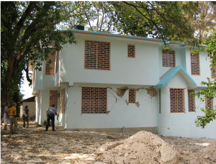
Figure 2: Newly constructed building which is a hybrid of reinforced concrete and CMU block.
