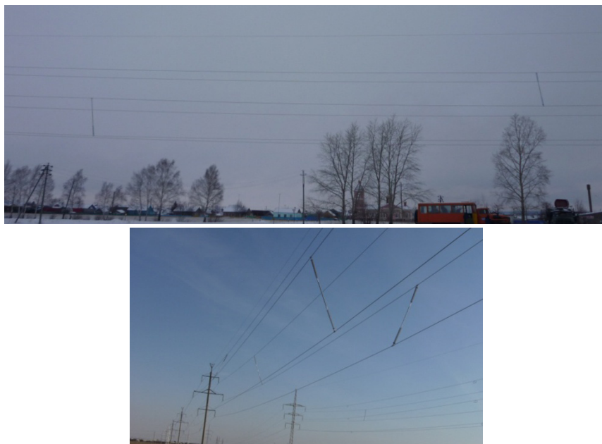
Figure 5: Interphase spacers on transmission line.
