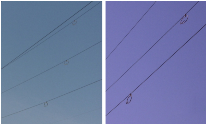
Figure 4: Counterweights on transmission lines.
