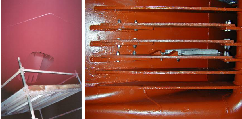
Figure 2: Picture of a Surface Ship seachest opening (left) with splitter bars removed and close-up (Right) with bars and sacrificial anode installed.
