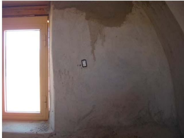
Figure 2: Sensor installed on the wall inside the building compartment.
