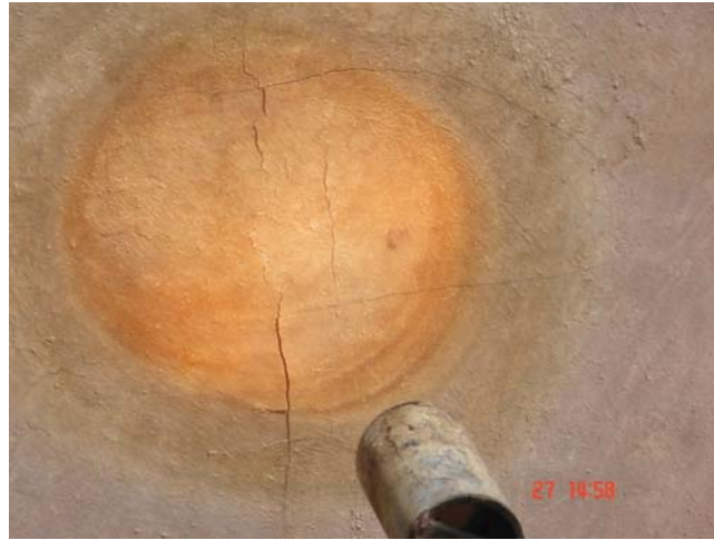
Figure 5: The cracks of the exposed area of specimen Mix C after 90 minutes.
