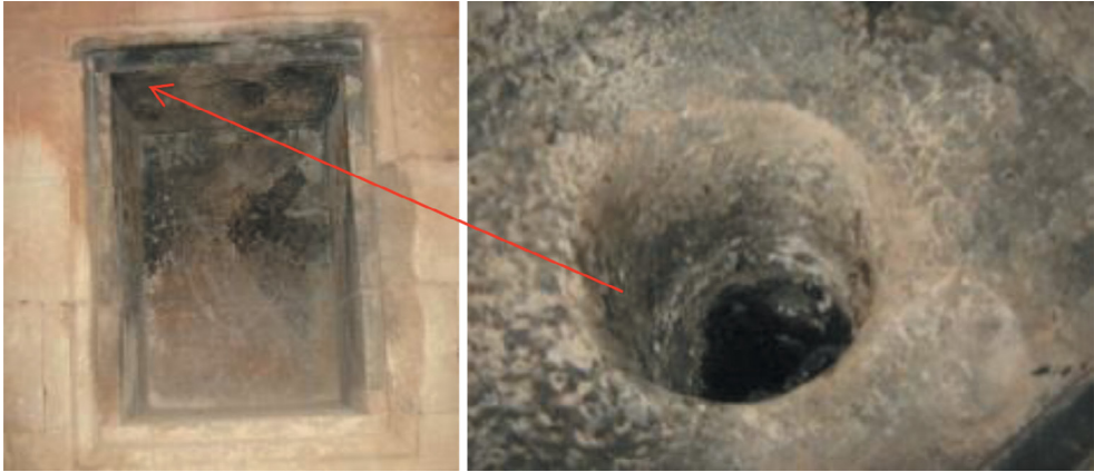
Figure 2: A niche (left) and its ventilation hole (right) on one of the walls in İshak Paşa Palace, used for candles (photo: author's archives, 2011).
