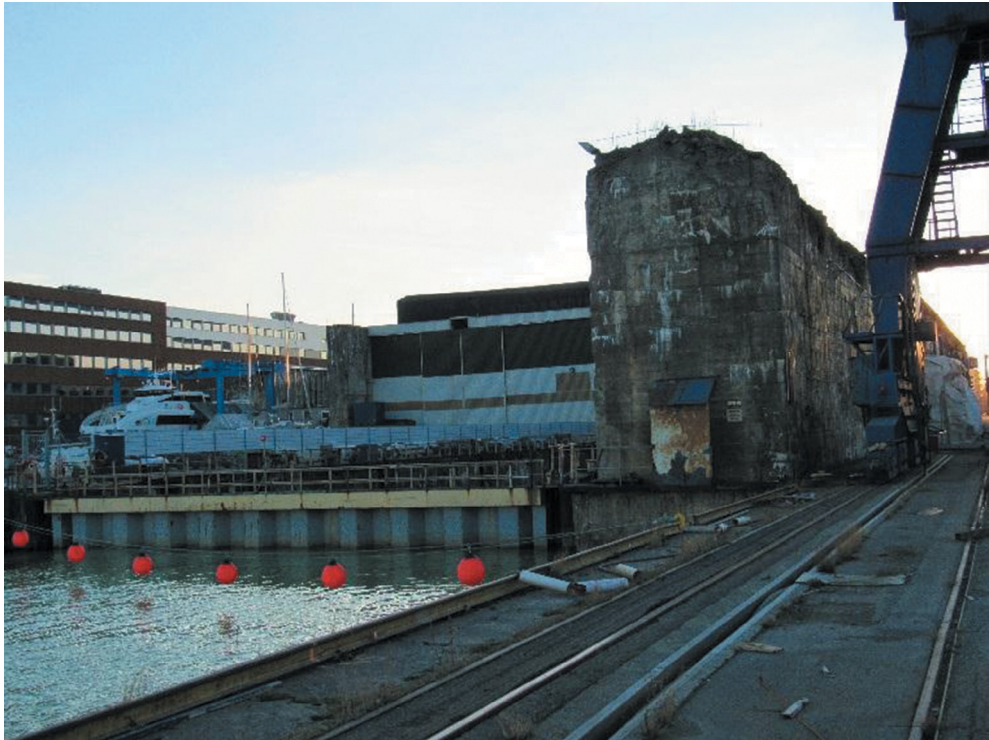
Figure 1: The never complete, partially demolished Dora II with the intact dock gates shut, January 2016. (Photo by S. Carstens.)
