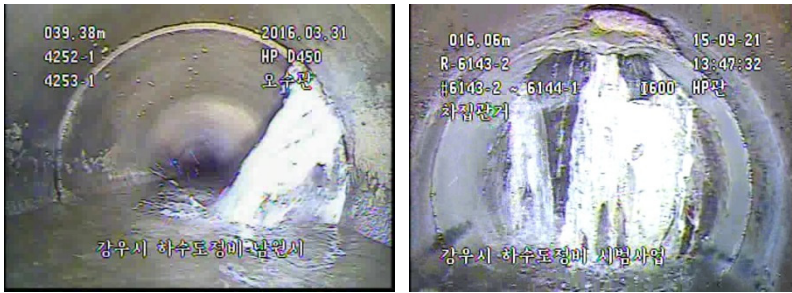
Figure 3: The pictures of internal interceptor sewer conditions in Nam-won.
