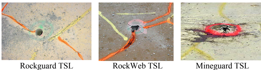
Figure 8: Limited radial damage about blastholes for TSL-only supported sites.
