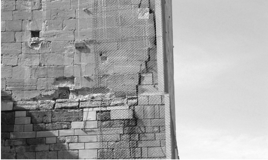
Figure 5: Tower of Sta. Maria de Alcocer : Damages caused by incompatible consolidation techniques manifest on matter in its appearance.
