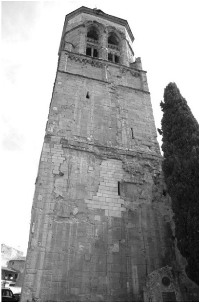
Figure 3: Tower of Sta. Maria de Alcocer consolidated with hidden techniques that can preserve documentary value of matter in its appearance.
