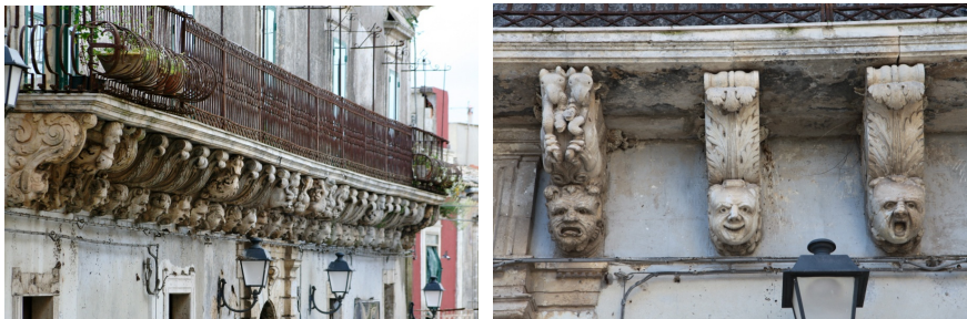
Figure 7: The balcony of Palazzo Judica Caruso. The longest of its kind, supported by 27 finely sculptured brackets.
