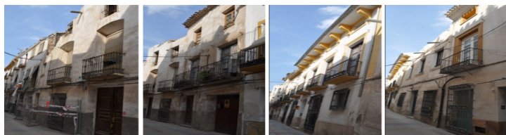
Figure 2: Buildings with heterogeneous damage in Cava Street.
