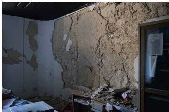
Figure 2: Office inside Colonia IX Maggio, abandoned after 2009 earthquake. (Source: E.G. De Leon.)
