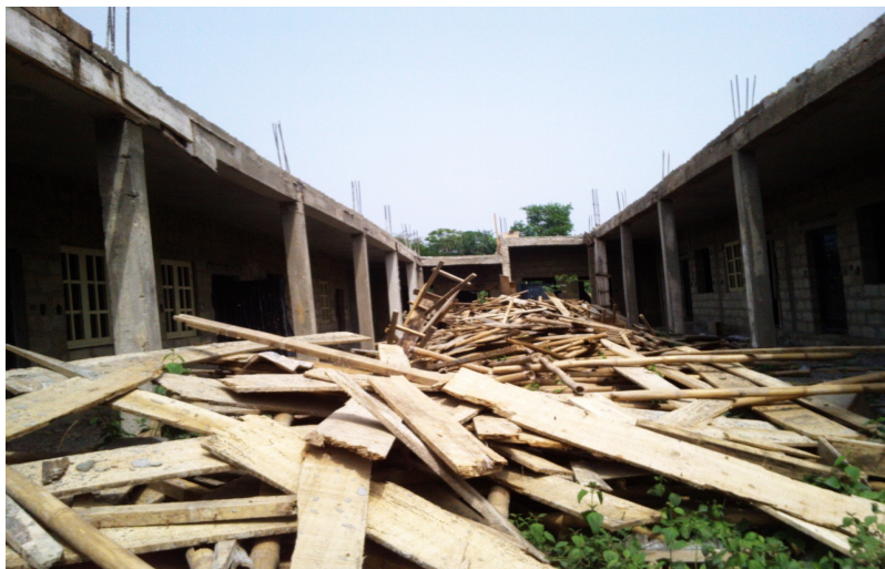
Figure 2: Wood and bamboo used as formwork after use on a construction site.
