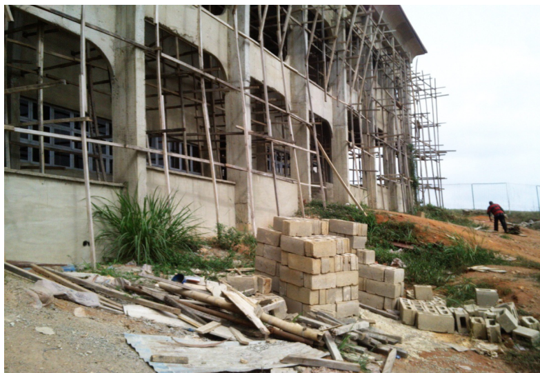
Figure 3: Construction waste: laterite soil from digging, sandcrete blocks, roofing sheets, laterite, bamboo and wood on a construction site.
