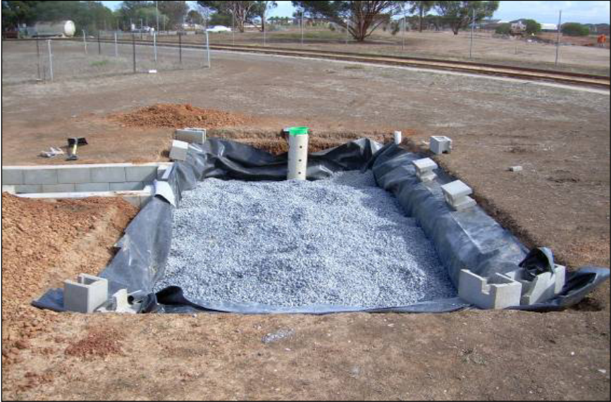
Figure 3: Perforated pipe for retrieving harvested stormwater.
