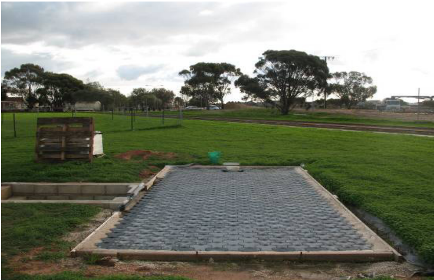
Figure 4: The completed UniSA prototype facility.
