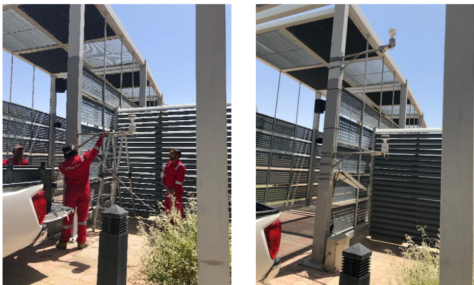
Figure 1: Site images of the installed sensor unit.
