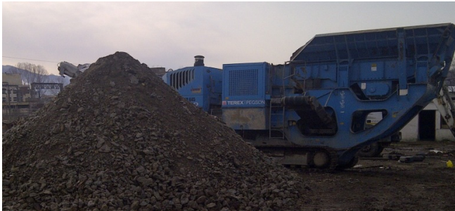
Figure 9: Crushing of the structural concrete locally.
