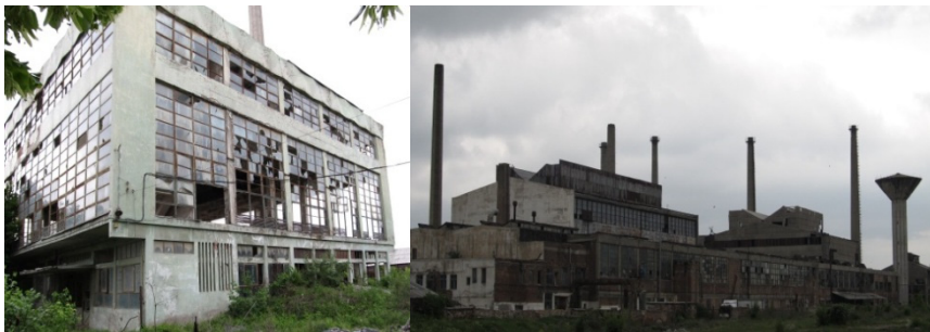
Figure 5: Structural skeletons in industrial areas in advanced deterioration.
