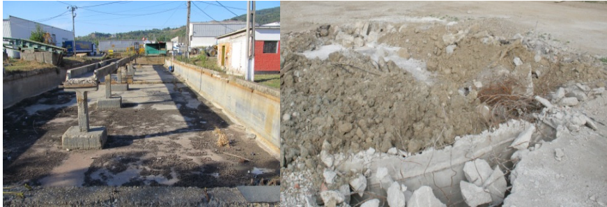
Figure 6: Structural skeletons in industrial areas in advanced deterioration.
