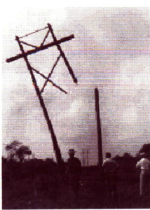
Figure 1: Damage due to strong wind [20].
