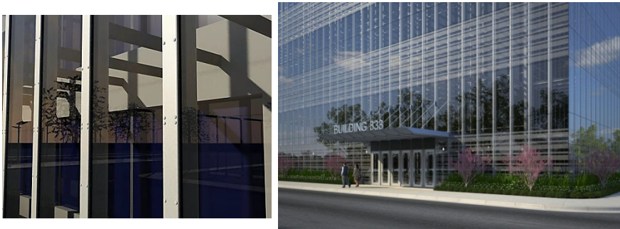
Figure 1: Polycarbonate blast-mitigating system retro-fit.
