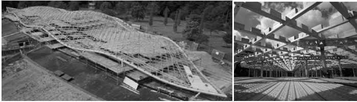
Figure 11: The Savill Garden grid shell was lowered into position gradually with vertically adjustable formwork [27].
