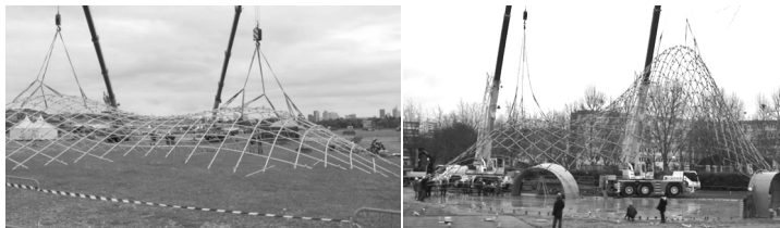
Figure 9: Crane erection of the Soliday Pavilion left [25, p. 10], and the Creteil Church right [26].
