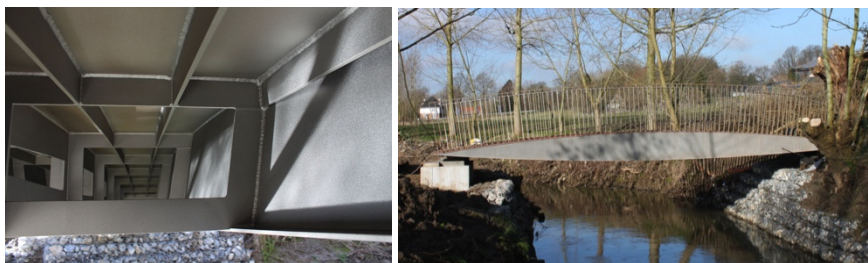
Figure 4: The inside of the braced caisson construction (left) and a view of the slender fish belly bridge deck (right).
