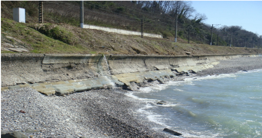
Figure 1: The condition of the coast protection structures at the Tuapse–Adler line. Dents in the bottom part of a seawall.
