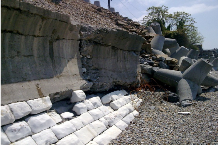
Figure 2: Seawall collapsed toward the sea. Yakornaya Schel Station.
