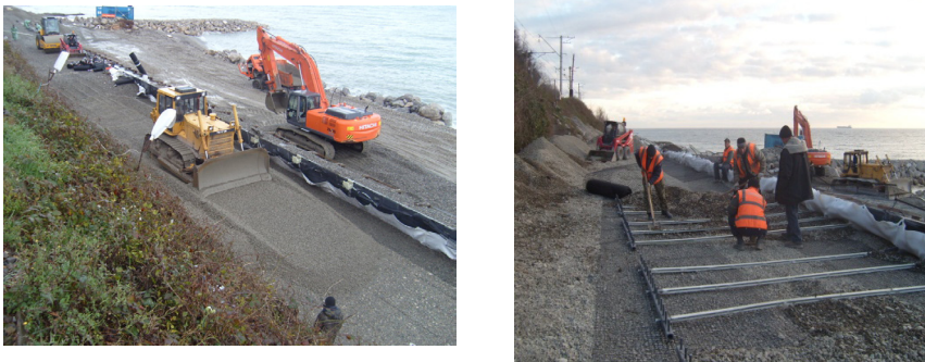
Figure 6: The layout of the Tensar SS-30 geogrid on the left, filling and grading of pebble with a fraction of 20-40 mm on the right.
