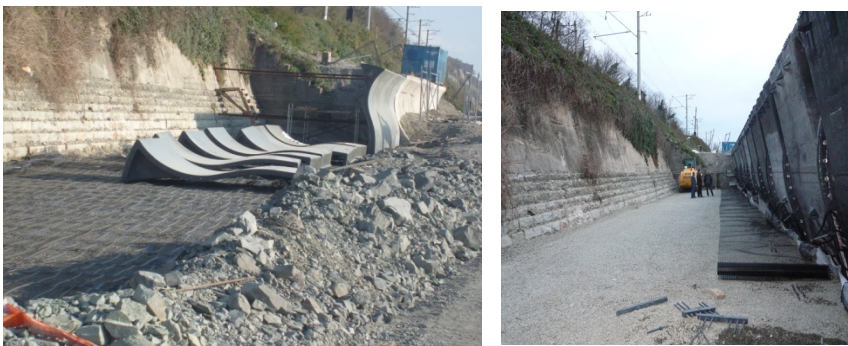
Figure 5: Fiberglass panels. The left-hand part shows installation of the fiberglass panels and the right-hand part shows the flange joints.
