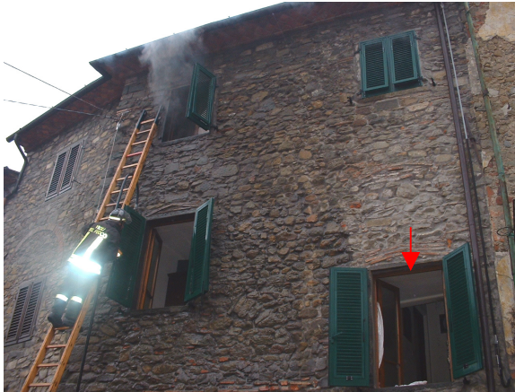
Figure 1: External view of the 2nd floor room originating the fire and of the window that vented out the backdraft flame (pointed by the arrow). All the pictures have been taken about one hour later the fire event.
