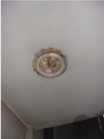
Figure 2: Detail of the 2 nd floor stairway lamp showing cover destruction.
