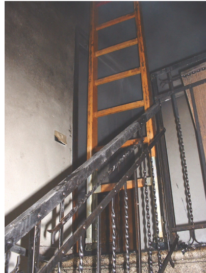
Figure 3: 2 nd floor stairway. The room originating the fire is on the left side.
