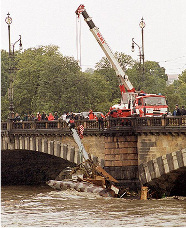
Figure 3: Accepted temporary measure - crane removing floating debris from bridge piers
