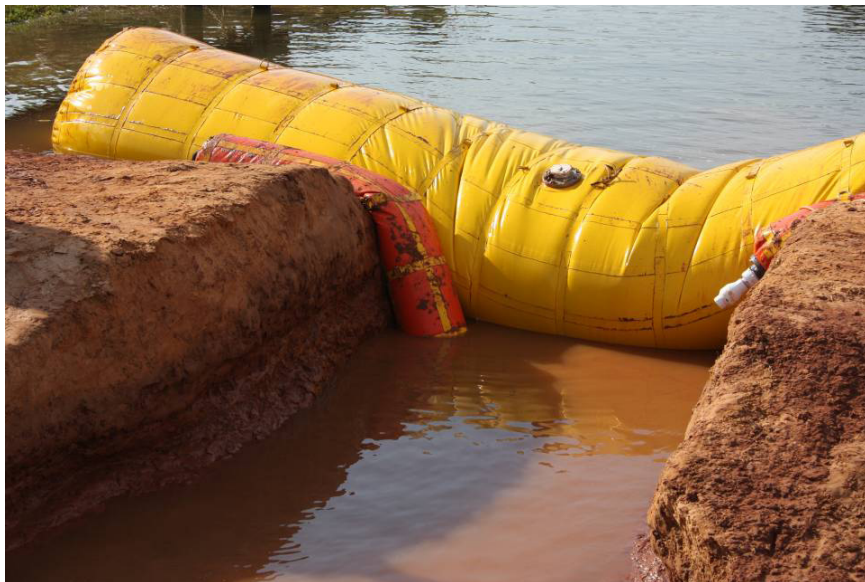
Figure 8: Sample deployment of deep-breach closure system including the addition of two small tubes along the upper edges of the breach opening which produced essentially zero-flow conditions through the breach.
