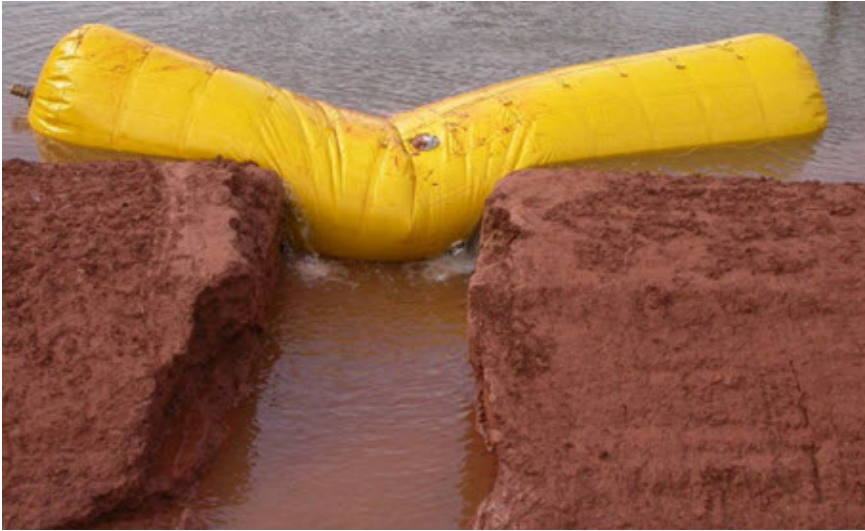
Figure 7: Sample deployment of deep-breach closure system, with a small residual flow still persisting along the upper edges of the breach opening.
