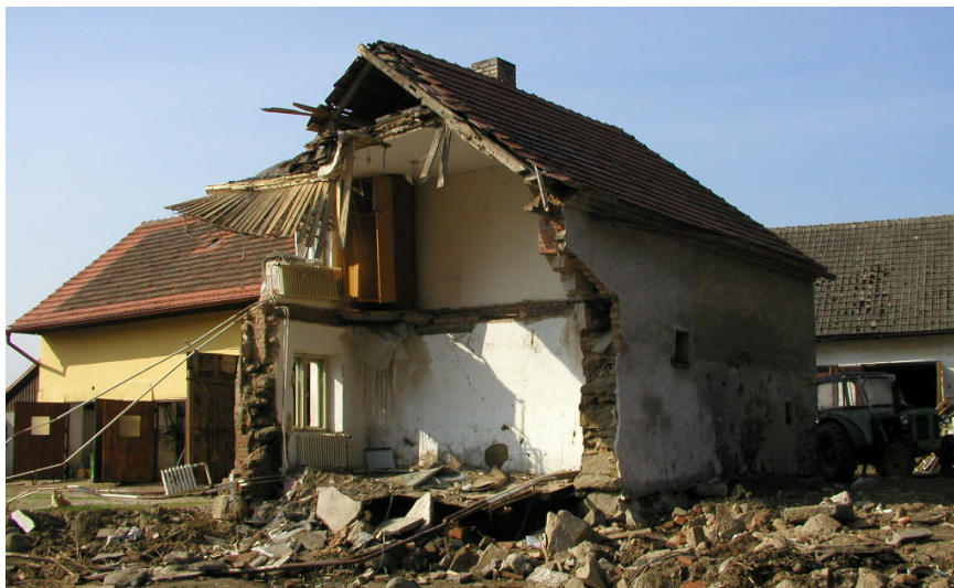
Figure 1: Failure of a structure with insufficient robustness.
