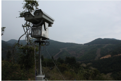
Figure 1: The cameras installed on a weather tight pan-tilt platform.
