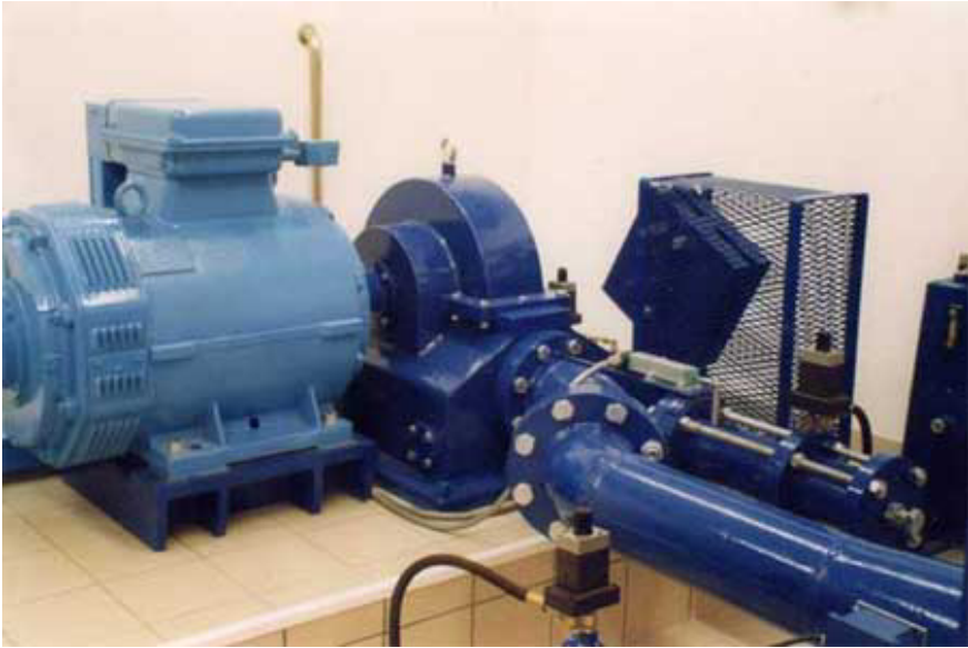
Figure 5: Pelton turbine installed on aqueduct with by-pass (tamanini).
