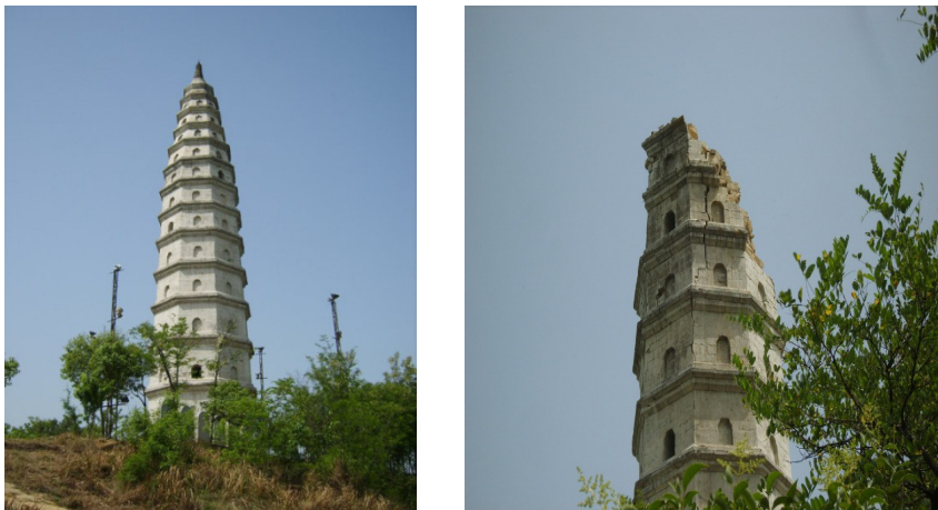
Figure 9: Laiyan pagoda (left: before the earthquake; right: after the earthquake).
