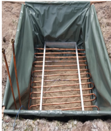
Figure 2: Ground copper pipe loop heat exchanger.
