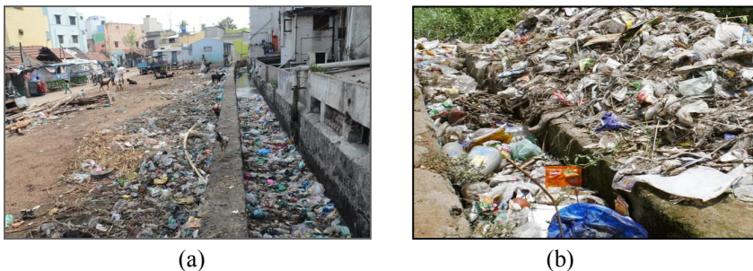
Figure 2: (a) Street dumping; (b) drainage dumping.
