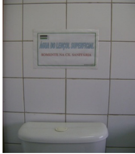
Figure 4: Notice regarding the use of recycled water in the bathrooms.
