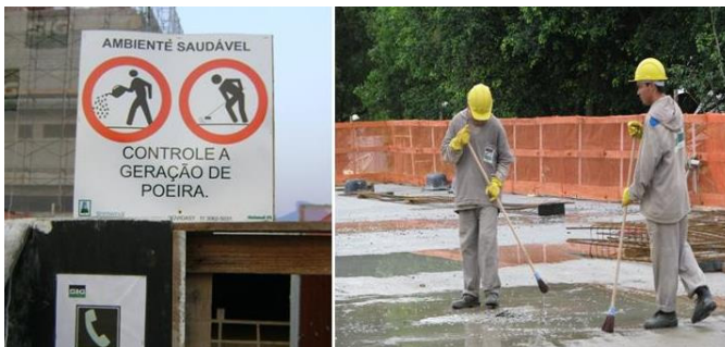
Figure 2: Control of sedimentation and sweeping of the construction site using rainwater and avoiding the generation of dust.
