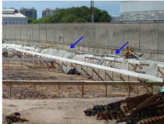
Figure 1: Embankments protected with screens to avoid erosion.
