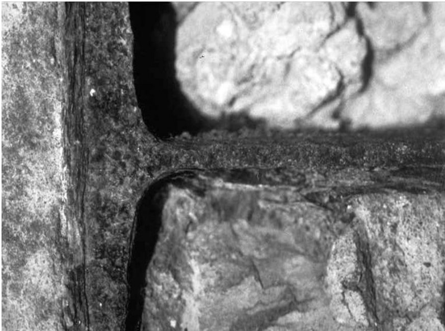
Figure 3: Corrosion of a masonry encased wrought iron beam.
