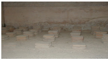
Figure 19: Heating system at the “thermae” from Augusta Raurica (October 2011).
