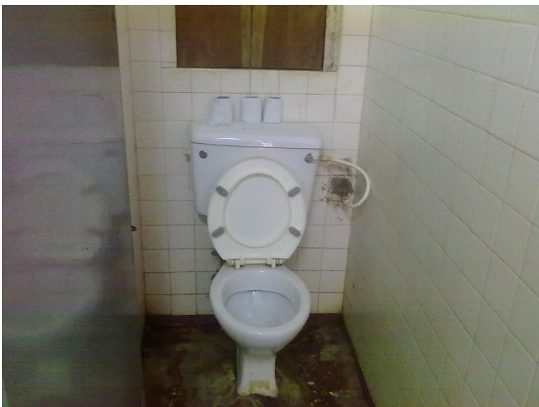
Figure 2: A case of a poorly maintained toilet in Fajuyi Hall, OAU, Ile-Ife.
