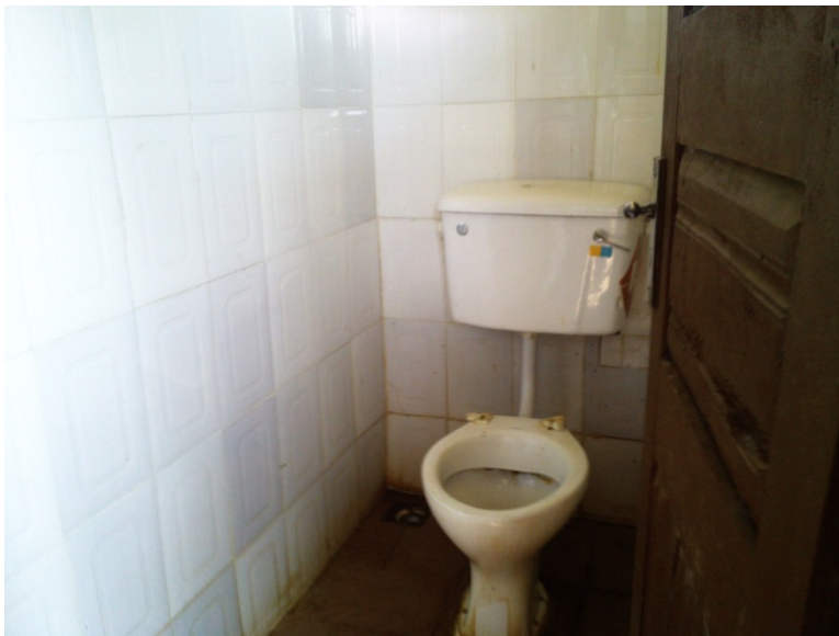
Figure 3: Non-functional water closet in Akindeko Hall, FUTA with defaced floor and a broken door.
