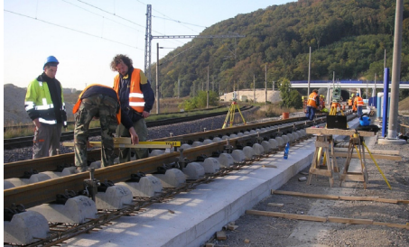
Figure 7: The tunnel Turecký vrch under construction with the view of the solid railroad RHEDA 2000 being built.
