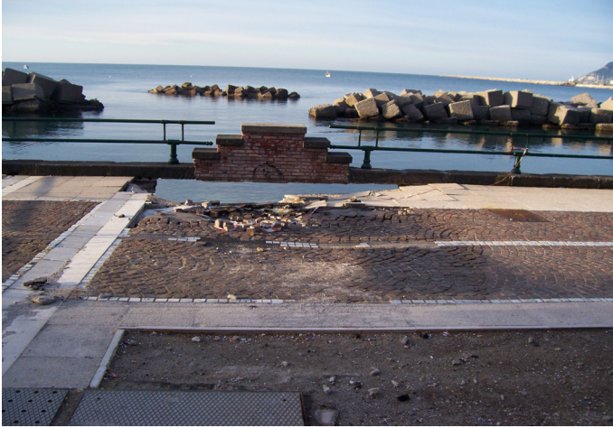
Figure 5: Damage to the waterfront of Salerno after the winter 2008 storms.
