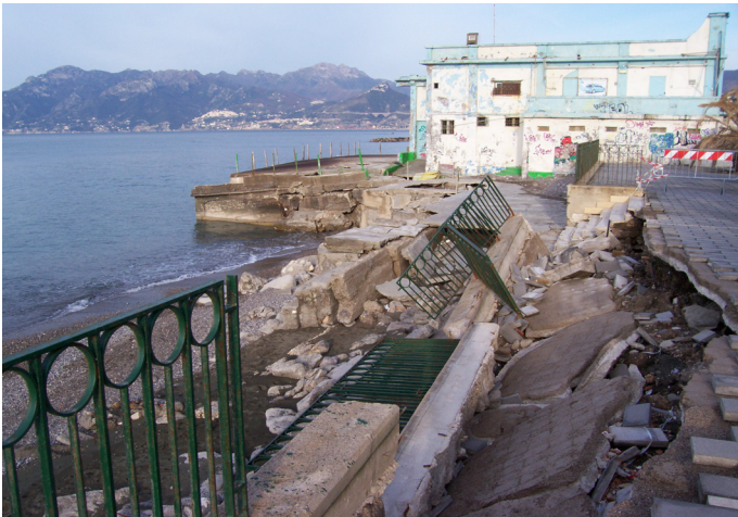
Figure 4: Damage to the waterfront of Salerno after the winter 2008 storms.
